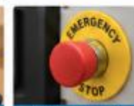
Know the emergency stop buttons.
